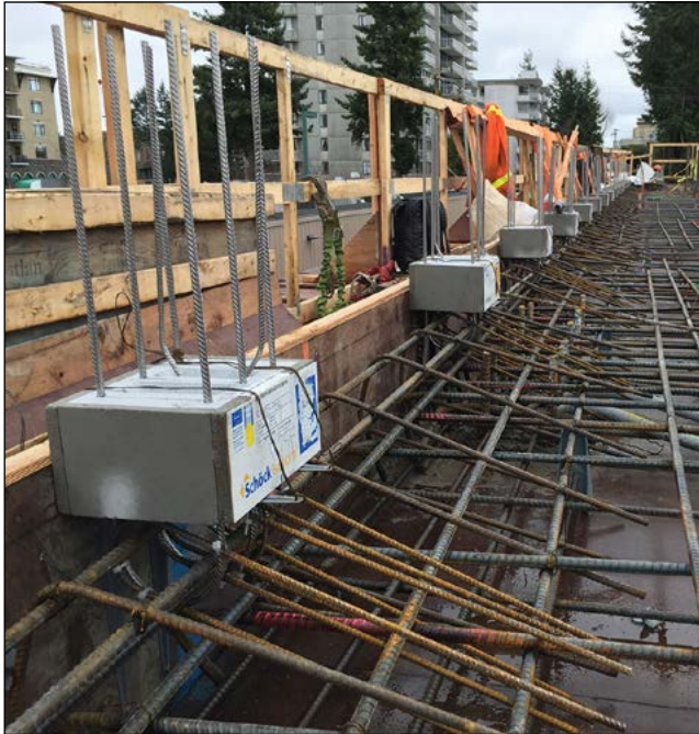
Figure 8: Isokorb® structural thermal breaks for parapets positioned against wooden parapet forms are tied into rooftop reinforcement before being cast in concrete.
